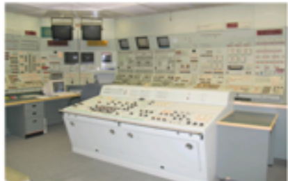
PLC Pickering Unit 5-8 Simulator
